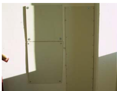
The holes in the breezeway stairs.
